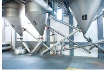
Gas purification processing units
