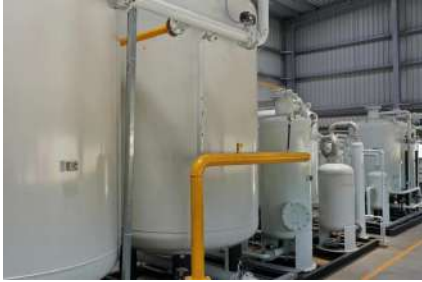
PSA purification vessels
