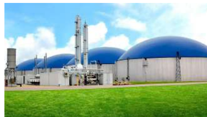
Anaerobic digestion dome tanks
