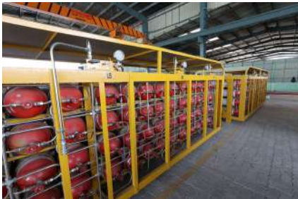
Compressed gas cylinder racks
