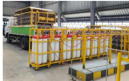
Gas distribution loading area
