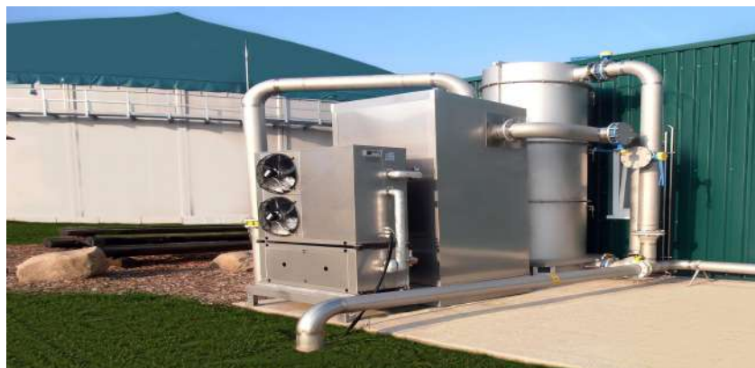
Gas processing & automation unit
