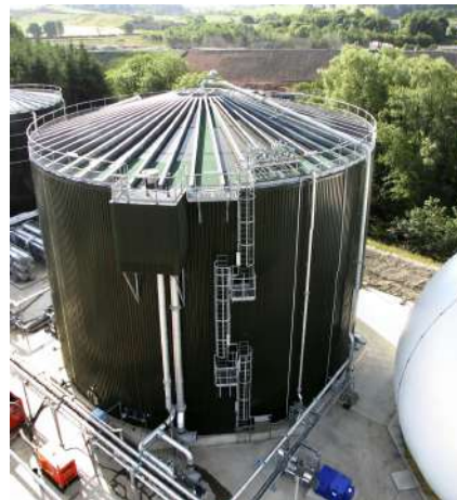
Large anaerobic digestion tank
